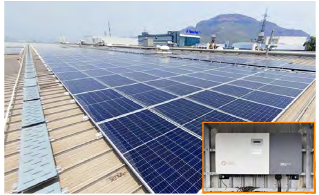
Tetra Pak Project, India 1MW
