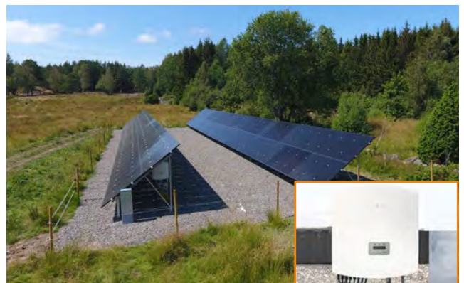
Västra Götaland, Sweden 43.3kW
