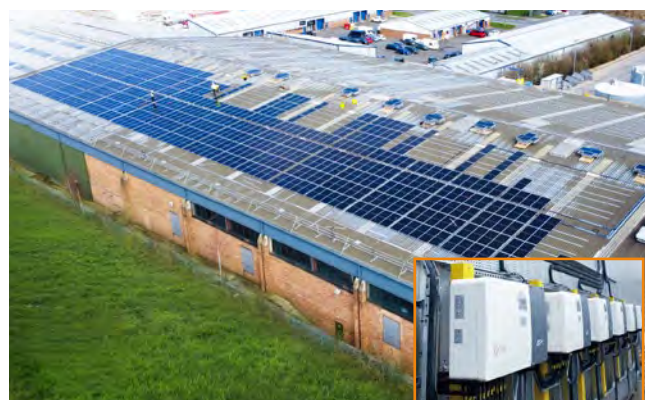
Faerch Plast Project, UK 2MW
