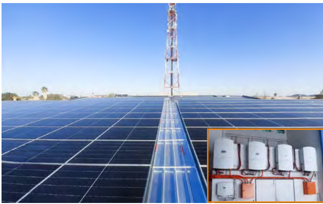
SolWorx Project, Namibia 272kW
