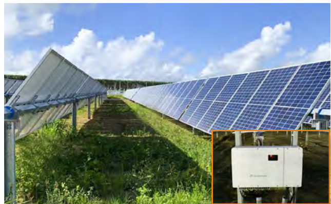
Vitoria Project, Brazil 2.5MW
