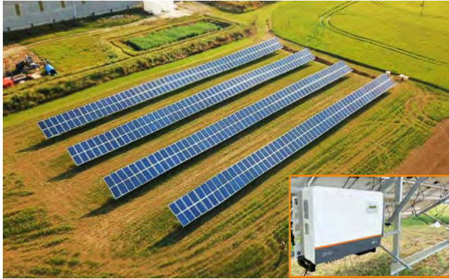
Lincolnshire, UK 140kW
