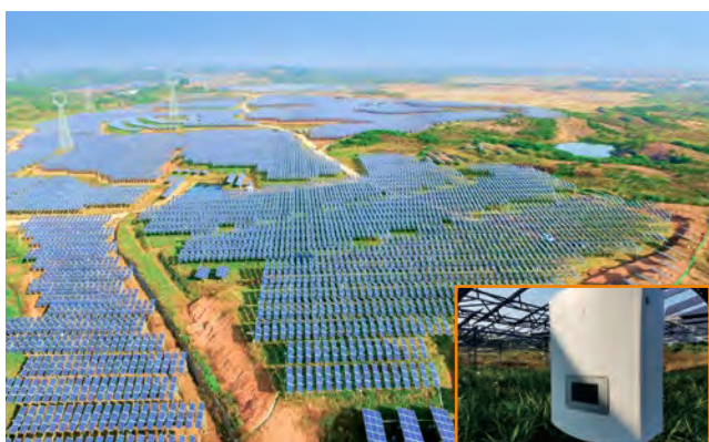
Zhejiang Hangbu Agricultural-photovoltaic hybrid PV plant 30MW
