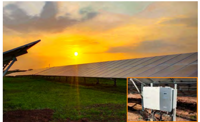
Grow Solar Project, India 10MW
